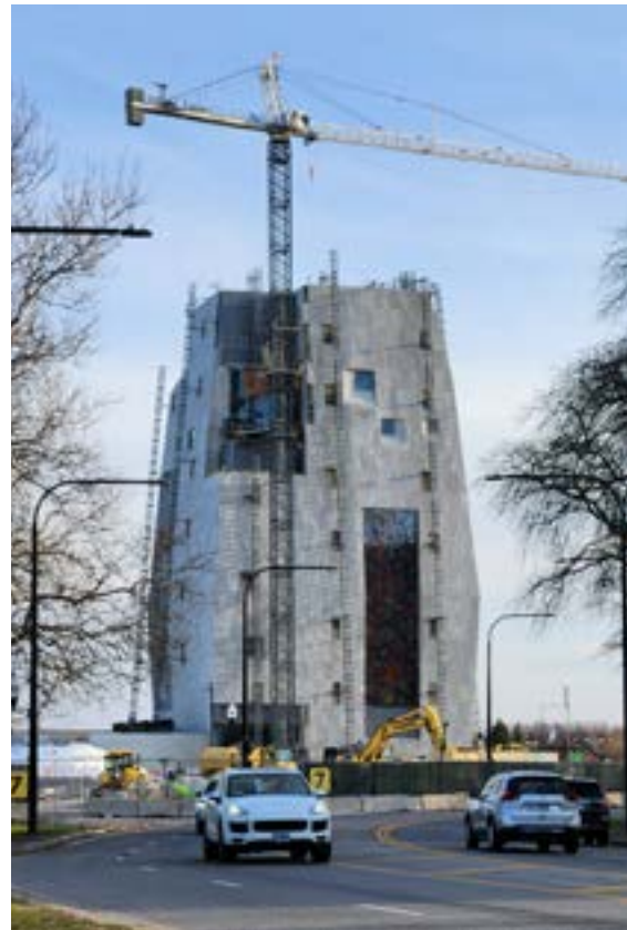
GEOptimize provided geothermal design support for the Obama Presidential Center in Chicago.
